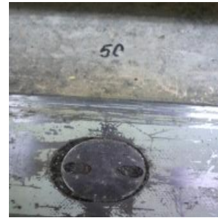
Fig. 4 Steel metal plate which marks the 50 m point of the geodetic base
